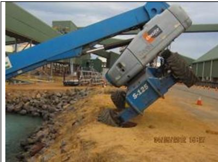
Photo 1 shows an incident where a Mobile Elevated Work Platform (MEWP) being operated close to a rock wall edge tipped due to instability of the ground surface.
