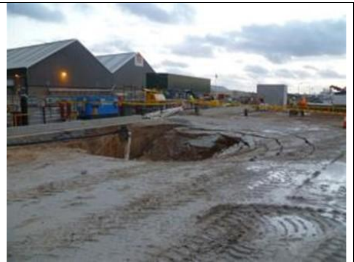
Photo 2 shows a sinkhole that appeared in the rail corridor.
